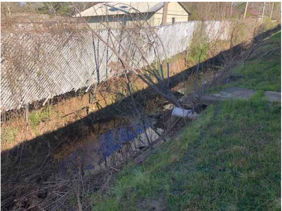
3 LOOKING NORTH DILAPIDATED FENCE TO BE REMOVED
