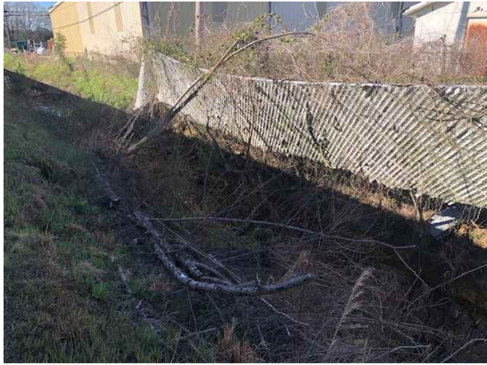
4 LOOKING SOUTH DILAPIDATED FENCE TO BE REMOVED
