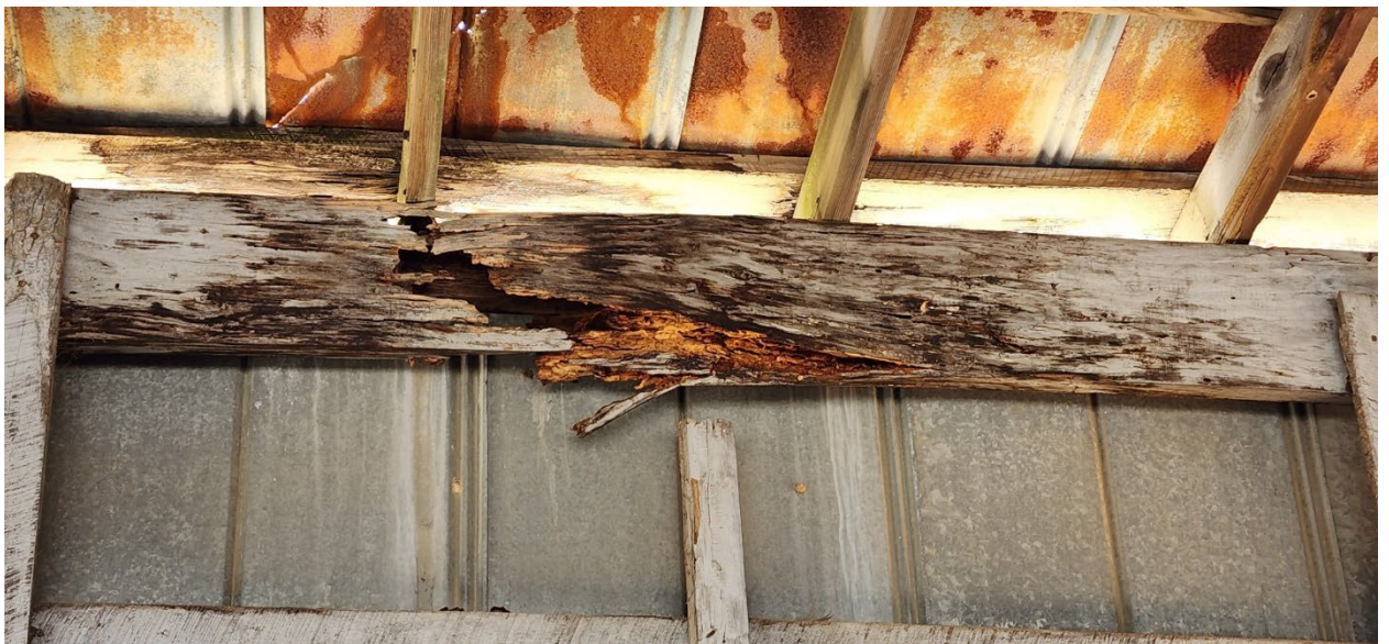
Photo 4 – Rotten Structural Member
