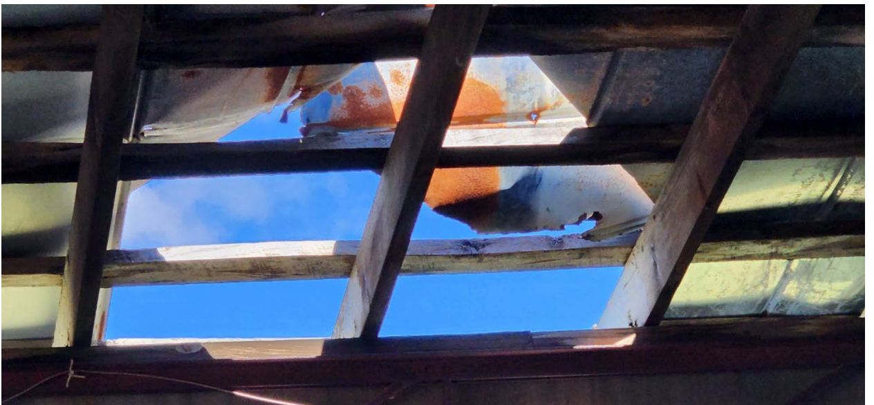
Photo 2 – Hangar Interior – Roof Damage
