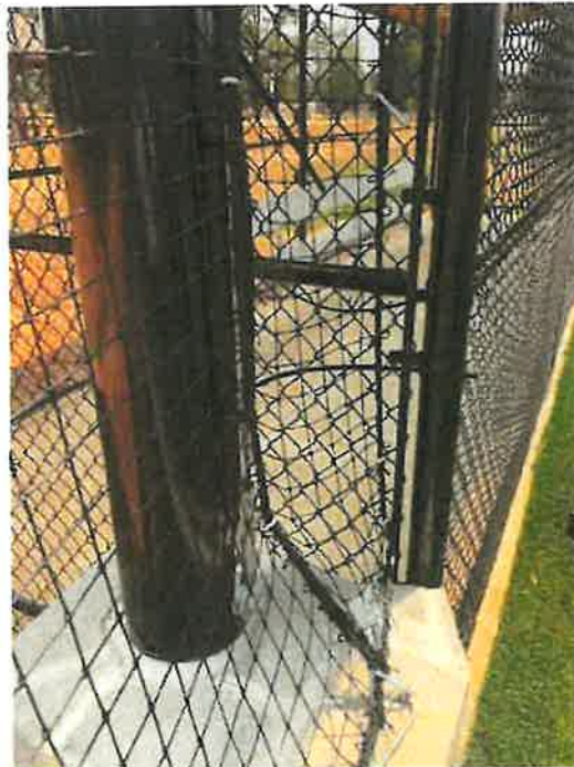
Photo 4 – Additional Gap Alignment and Closure Needs, Trim Zip Tie Excess.
