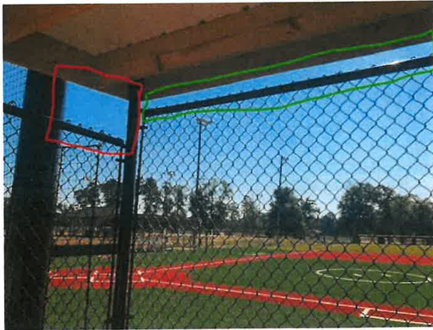
Photo 12 – Top Rail To Be Adjusted To Prevent Balls From Entering The Dugout, Typical All.
