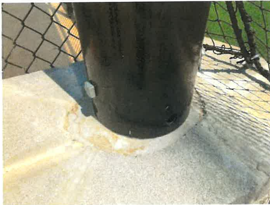
Photo 13 – Cover / Enclose Hole to Avoid Future Wasp Nest, Typical All Poles. Fill Expansion Space To Be Flush With Top of Block To Avoid Water Ponding, Typical of All Poles.
