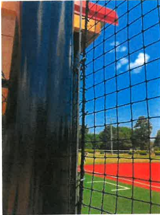
Photo 3 – Need Additional Tie to Close Vertical Gap in Netting, Typical All Corners.
