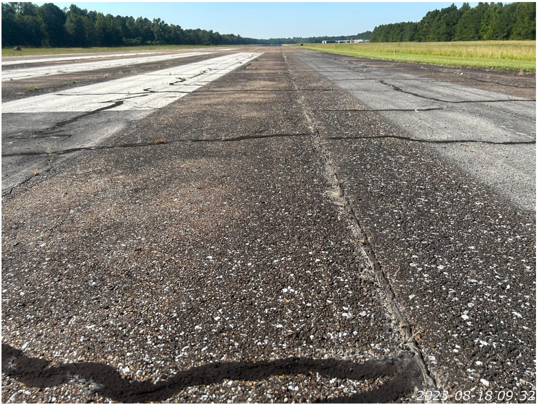
Photo 2 – Oxidation and Block Cracking in Runway Pavement
