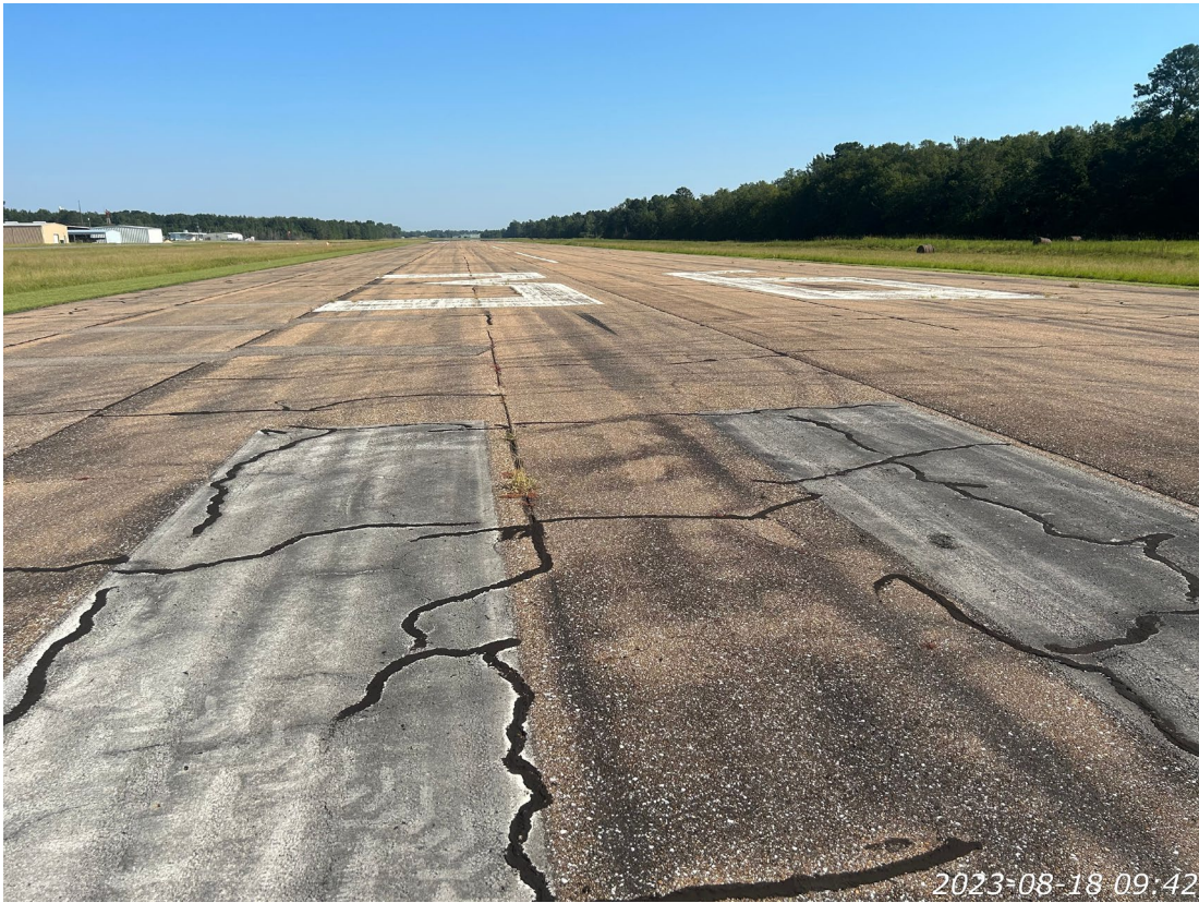
Photo 8 – Block Cracking in Runway Pavement
