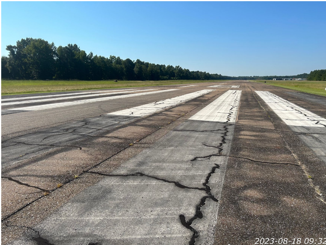
Photo 1 – Oxidation and Block Cracking in Runway
