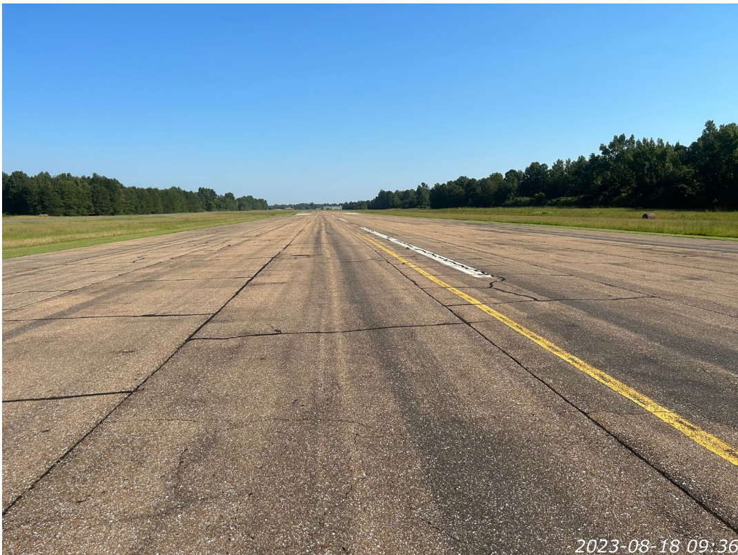
Photo 5 – Block Cracking in Taxiway Pavement
