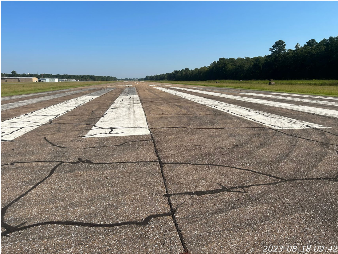
Photo 7 – Block Cracking in Runway Pavement
