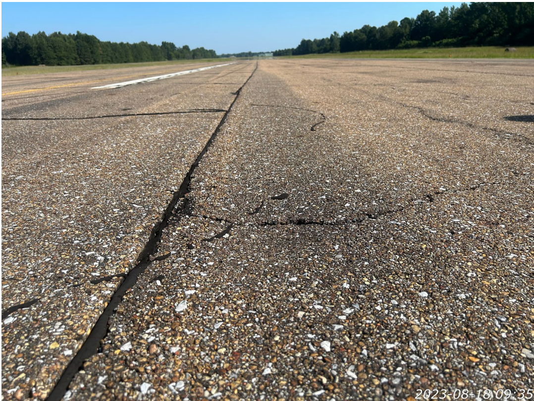
Photo 3 – Oxidation in Runway Pavement
