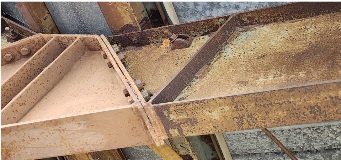
Photo 8 – Corrosion on Structural Steel
