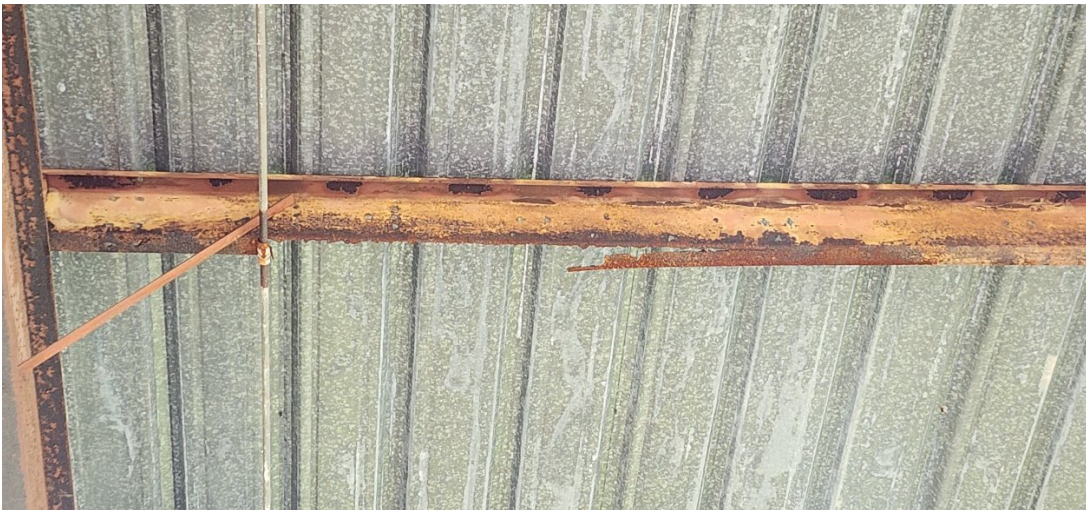
Photo 5 – Structural Member Section Loss/Corrosion
