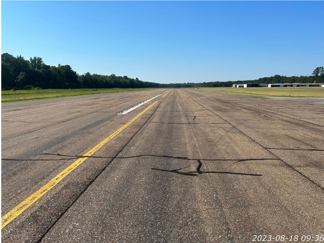
Photo 4 – Block Cracking in Runway Pavement
