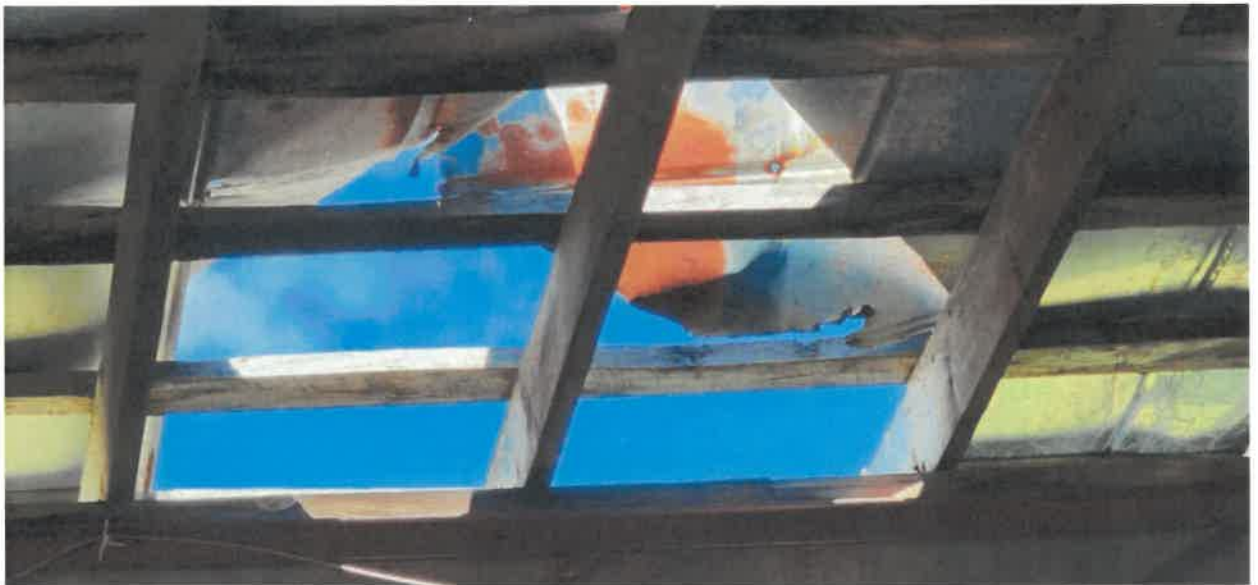
Photo 2 – Hangar Interior – Roof Damage
