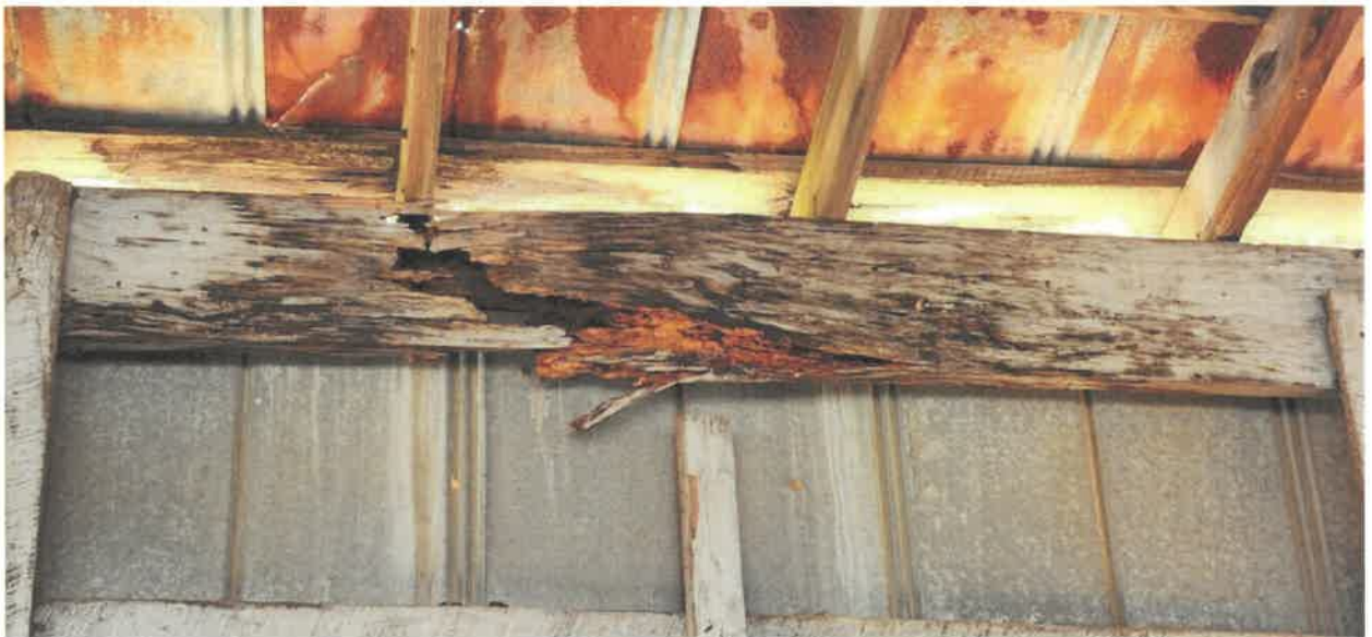
Photo 4 – Rotten Structural Member
