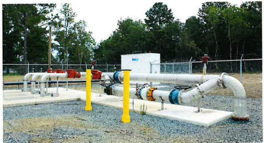
Jordan Road Pump Station, Jackson County, MS
