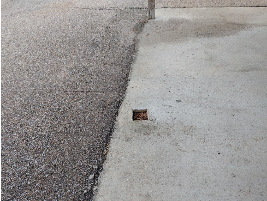
5. Displaced column location on the East side of the Market.
