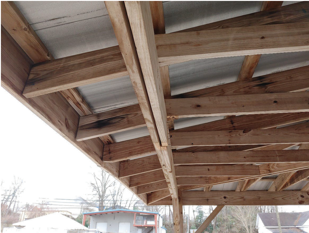
4. Displaced column location on the East side of the Market.
