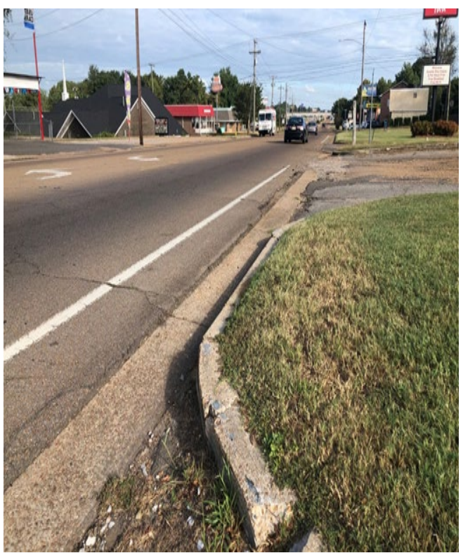
NO SIDEWALKS AND ACCESS ISSUES Looking North on East Side of 5 th Street - NOTE THE WORN GRASS FROM PEDESTRIAN USE -
