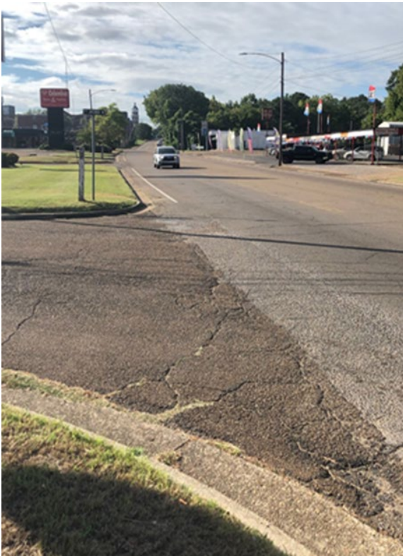
NO SIDEWALKS OR CROSSWALKS Looking South on 5 th Street @ 7 th Ave.
