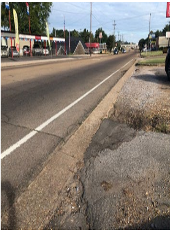
NO SIDEWALKS AND ACCESS ISSUES Looking North on East Side of 5 th Street
