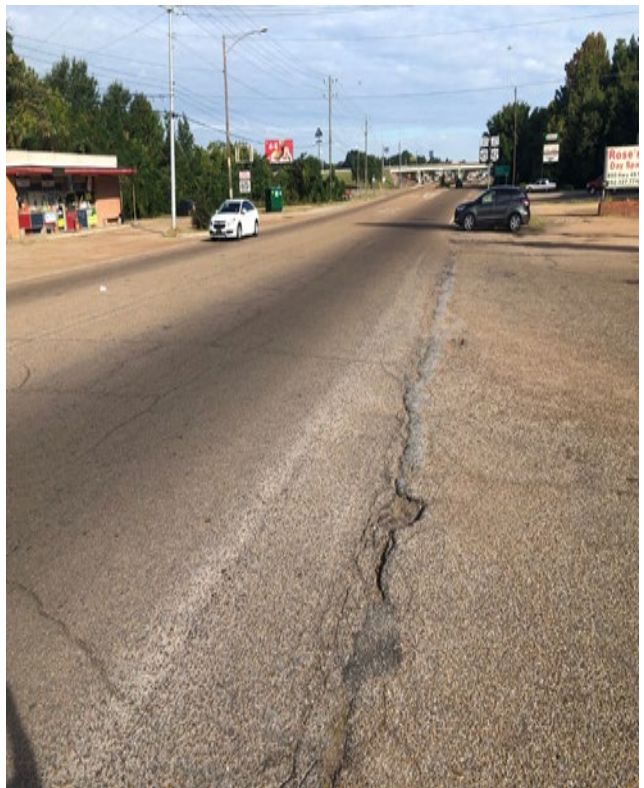
NO SIDEWALKS AND ACCESS ISSUES Looking North on East Side of 5 th Street
